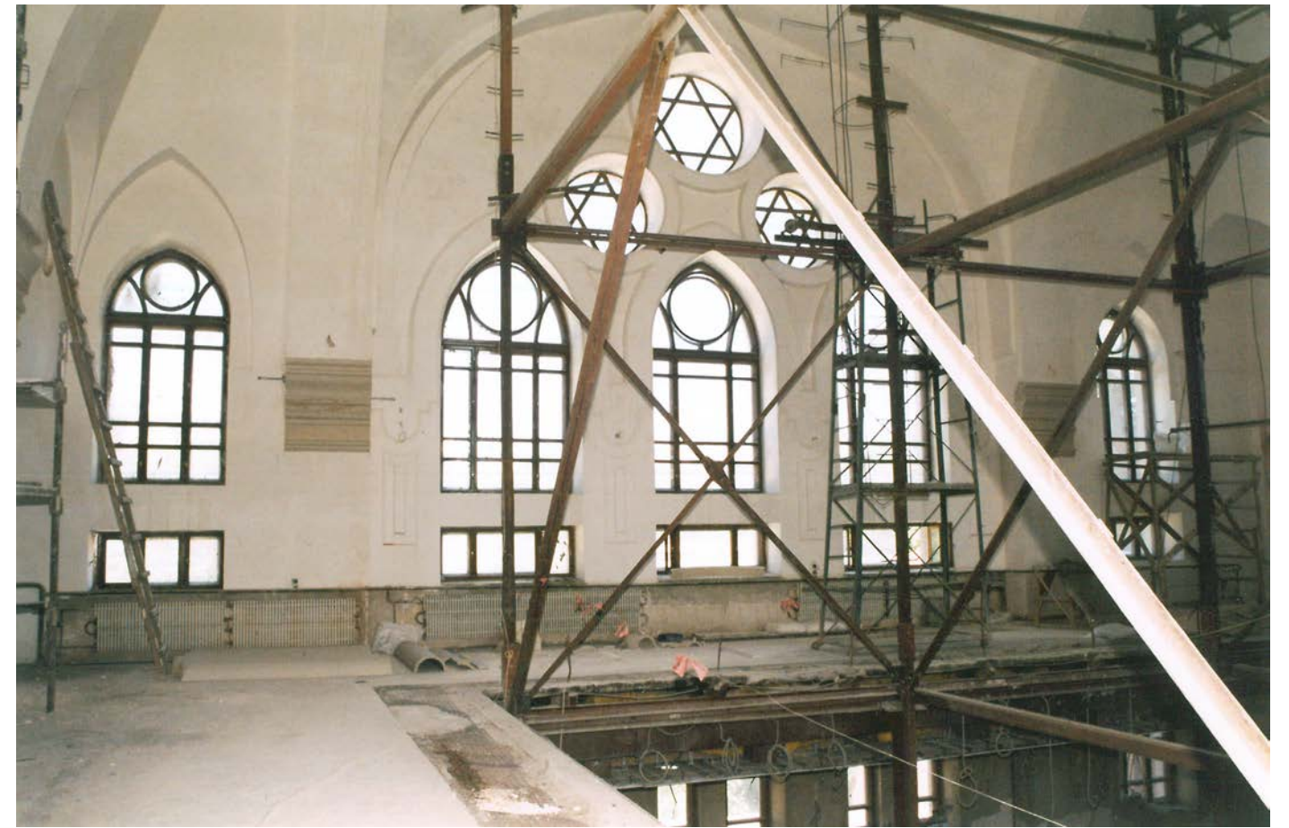
The Prayer hall of the synagogue under reconstruction. The end 1990s and early 2000s. Photo by E. Kotlyar
