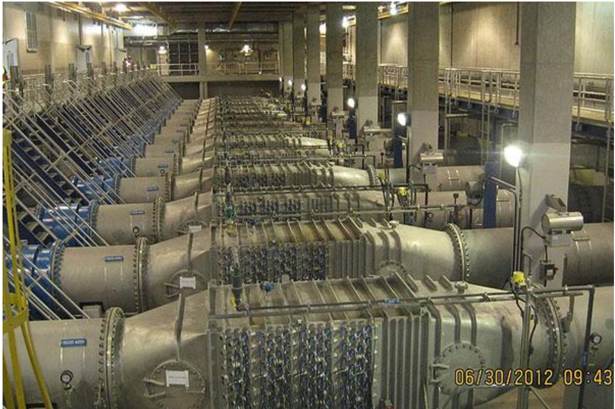
Figure 7 Catskill UV Treatment Plant 27
